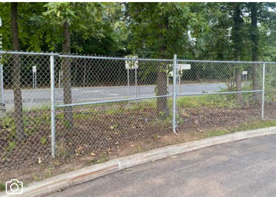
Before and After: Fence repairs and brush removal at Gaffney Elementary School.
